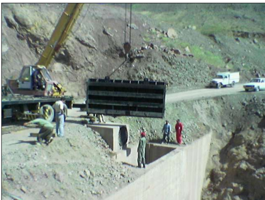
DIVERSION TUNNEL GATE
