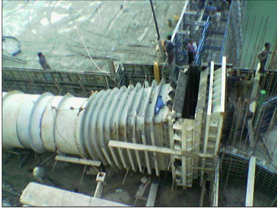
BOTTOM OUTLET EQUIPMENT
