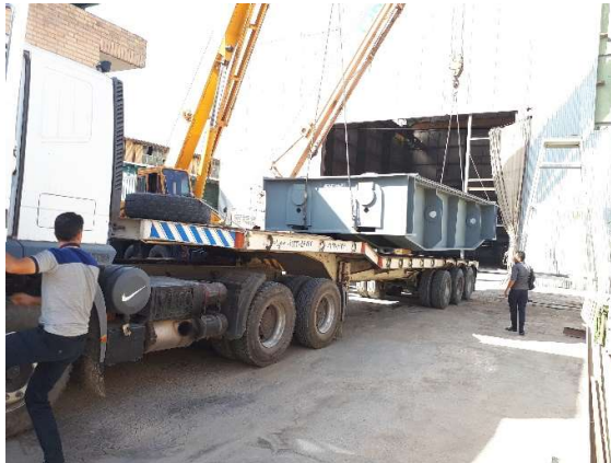
Khersan Dam Diversion Gate
