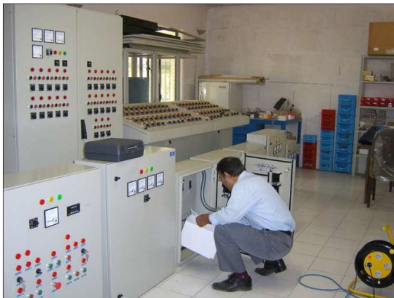
CONTROL ROOM EQUIPMENT
