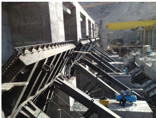
RADIAL GATE in OPERATION
