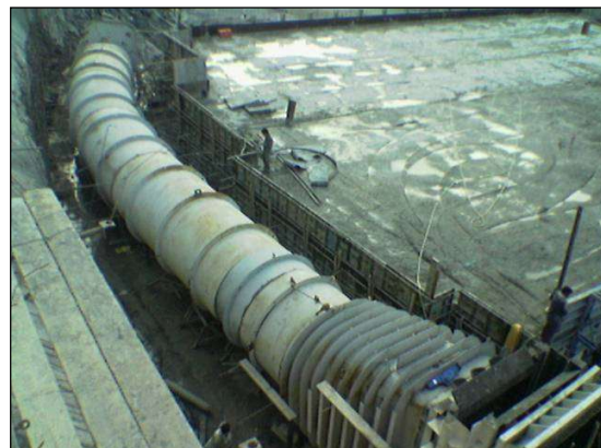
BOTTOM OUTLET EQUIPMENT
