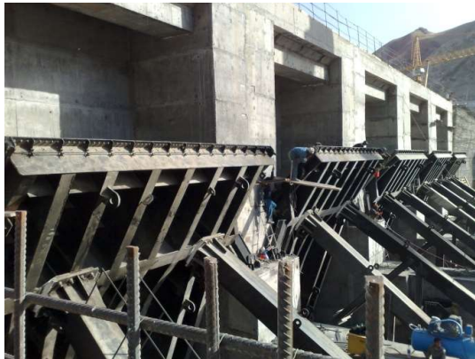
RADIAL GATE in OPERATION
