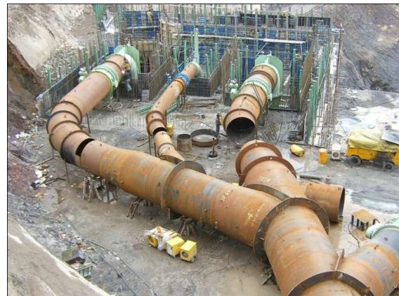
OUTLET PENSTOCK & VALVES
